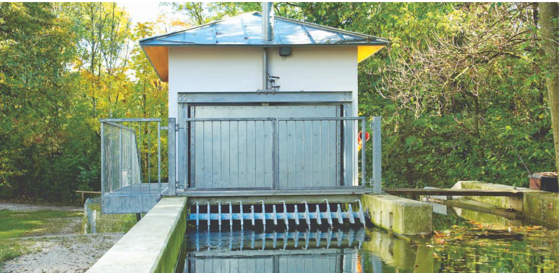
Complete equipment package • Inlet screen with automatic hydraulic sluice gate (Above) • High efficiency gearbox with generator (Opposite Page)
