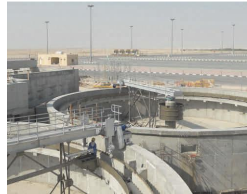
Stainless Steel Clarifiers at STP, Doha, Qatar
