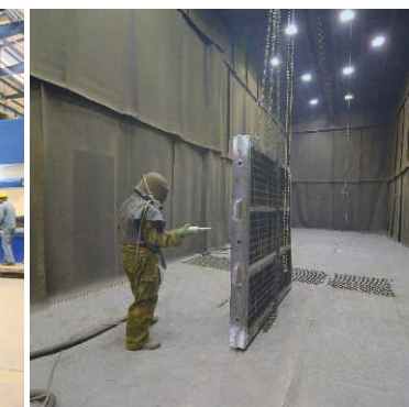
Shot Blasting Room (24 x 6 x 6m)
